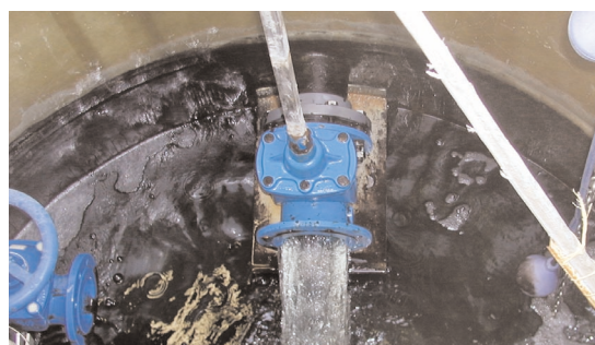
Drainage outflow in the collection sump
