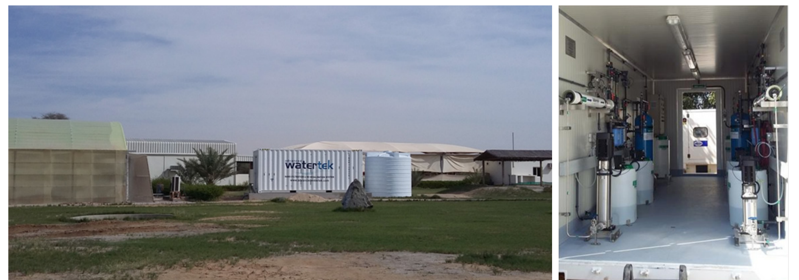
Installation of RO and Nano units at ICBA
